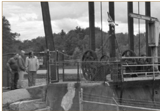
▲ Inspecting the Pepperell Hydro station's inlet gate are, from left, Wilmington CAB member George Hooper, RMLD General Manager Vinnie Cameron and RMLD Commissioner Phil Pacino. The inlet gate regulates the flow of water to the powerhouse, which spins turbines, which generate electricity.
