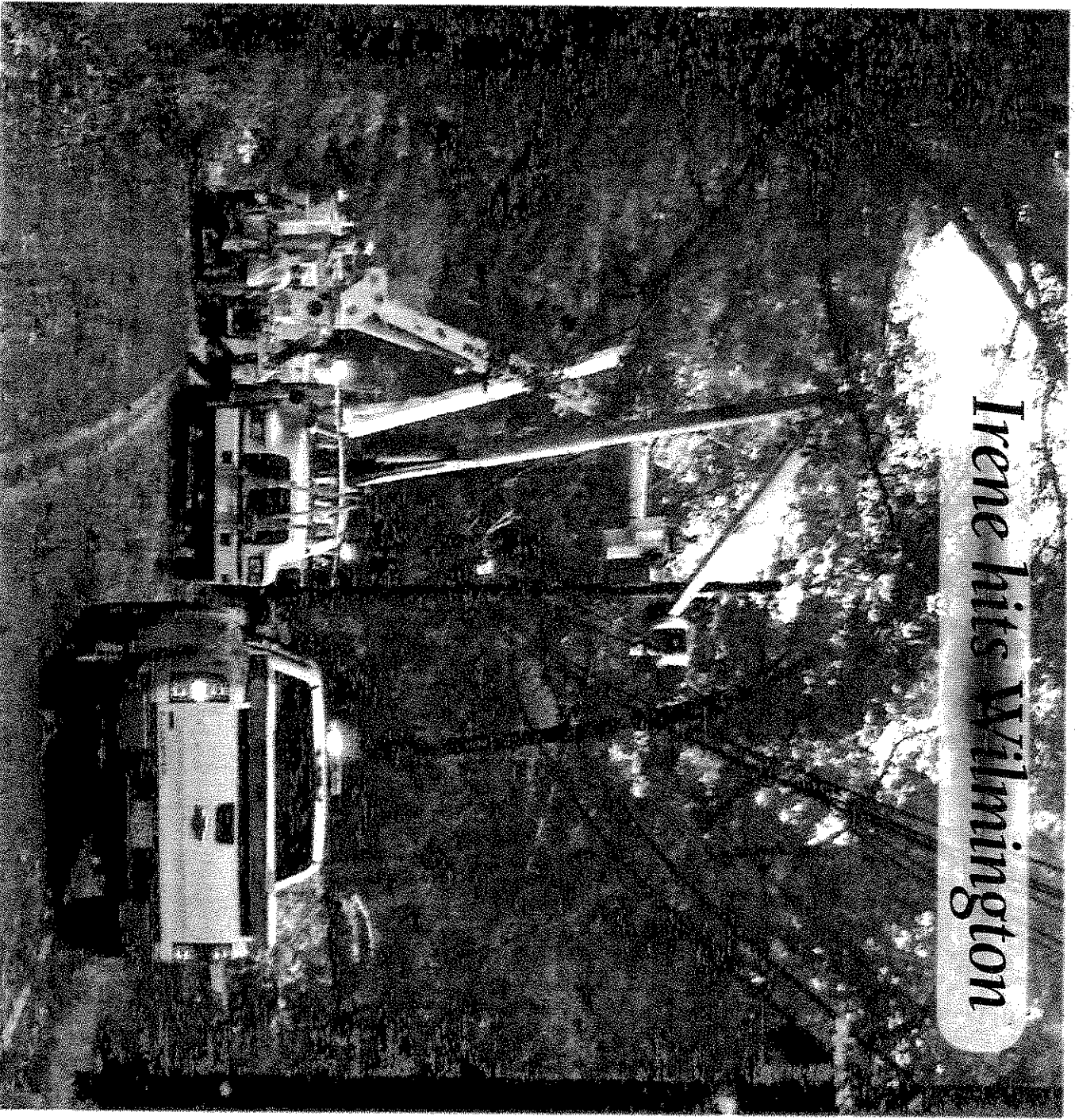
Reading Light crews were on West Street Sunday afternoon repairing wires that were torn down by falling limbs from Hurricane Irene.
